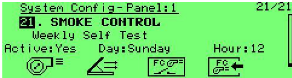
Screen 66 System configuration – Smoke control test settings
